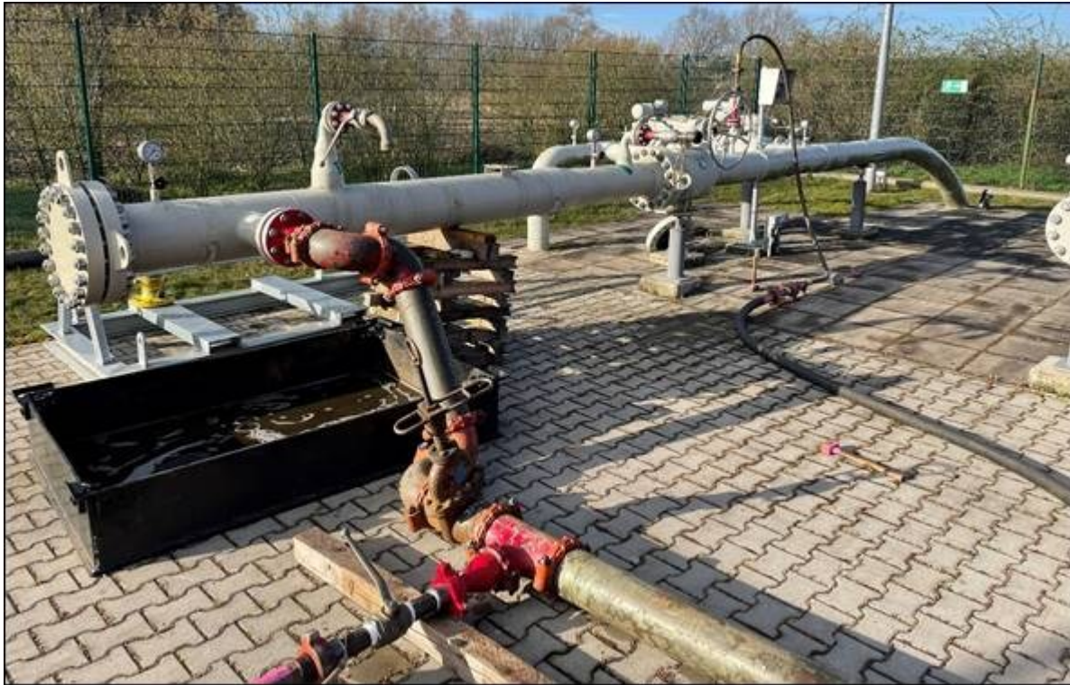
Abbildung III.6.3: Sendeschleuse Station Holthausen II
