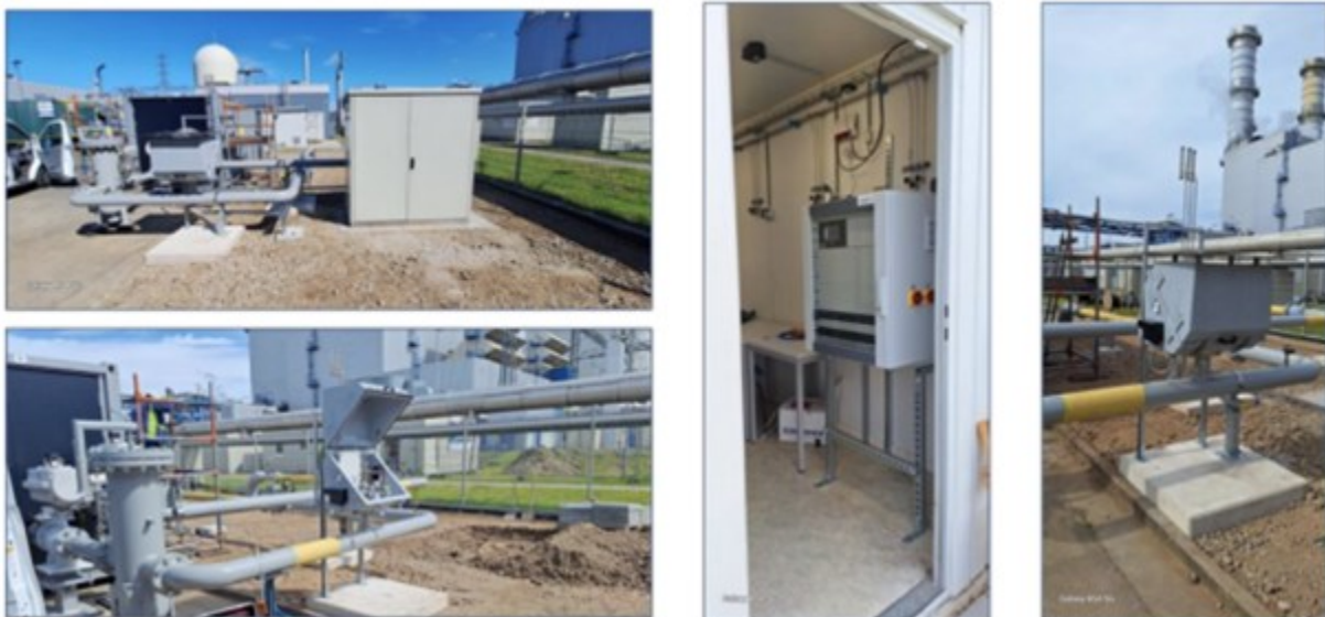
Abbildung III.3.6: MGC hydrogen -Installation in Lingen
